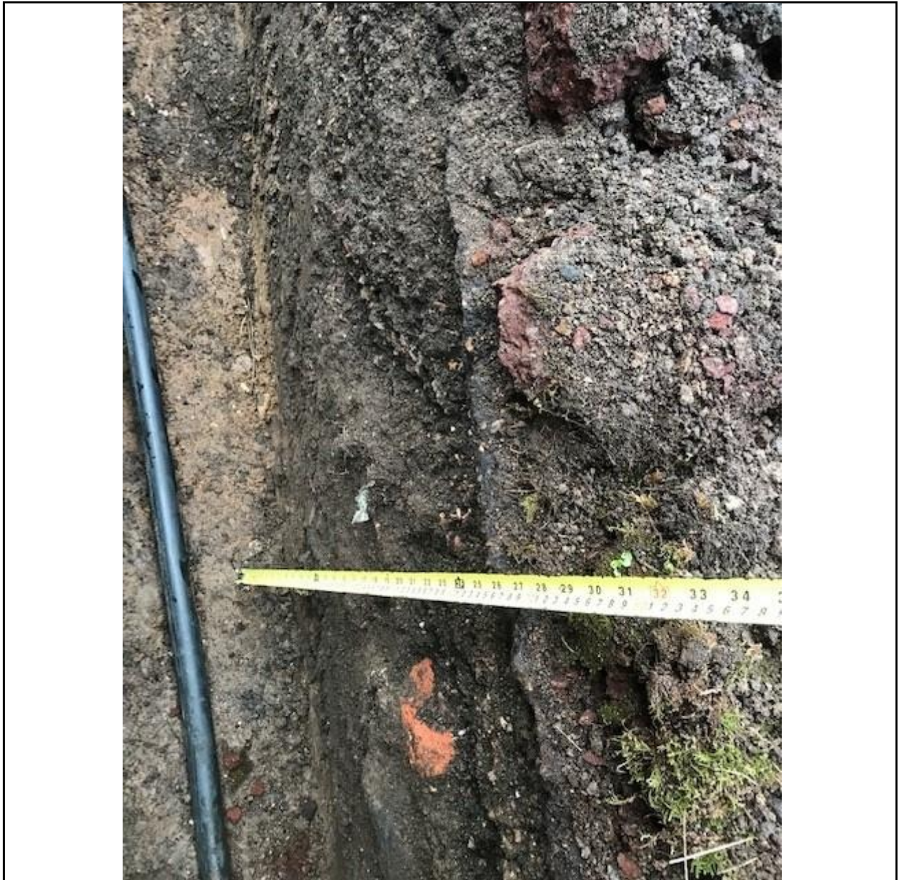
Figure 4. Site owners photo from trench dug across site for electrical works in January 2024.
