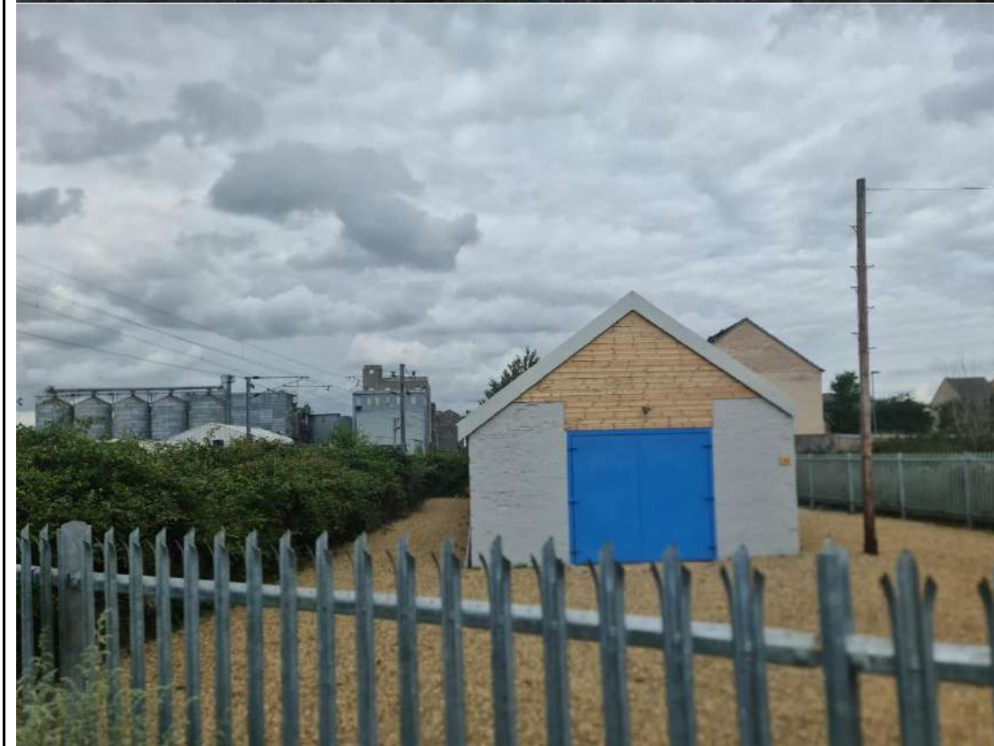
Photograph 4: (Above(a)) Former Garage, previously overgrown but looks recently cleared and fenced (December 2022) (Below(b)) Renovation works undertaken to the structure (20/07/23)
