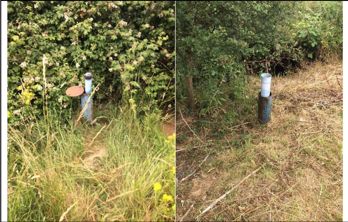
Photograph 7 a&b: LFG 4 & GW1 showing displacement of casing July 2014
