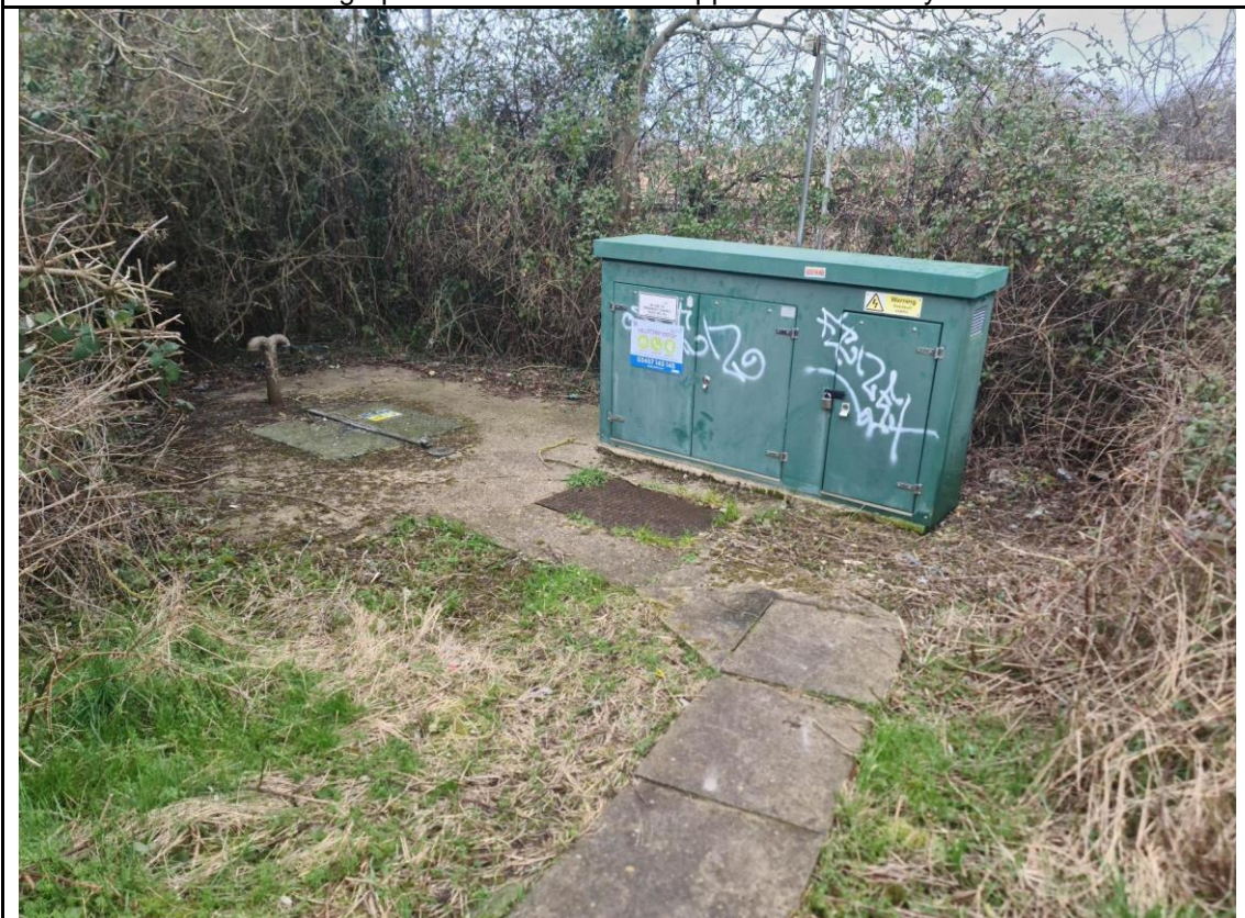
Photograph 2: Sewage and electrical infrastructure at the south of site.
