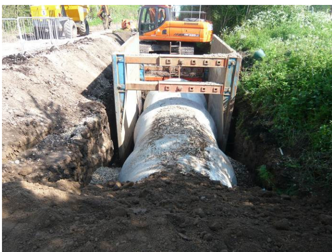
1.8m internal diameter concrete pipe
