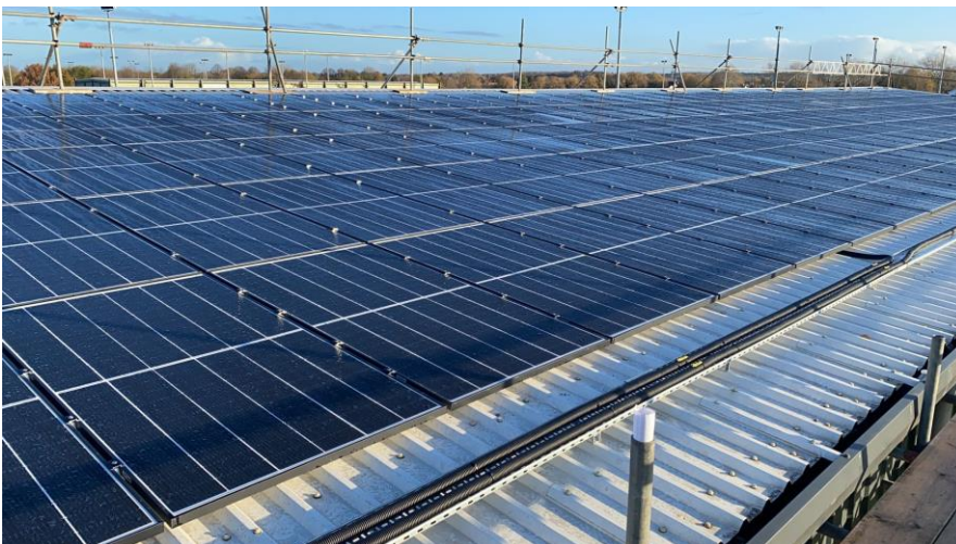
Figure ES 2 – Solar (Photovoltaic) Panels Installed at Lynnsport Leisure Building
