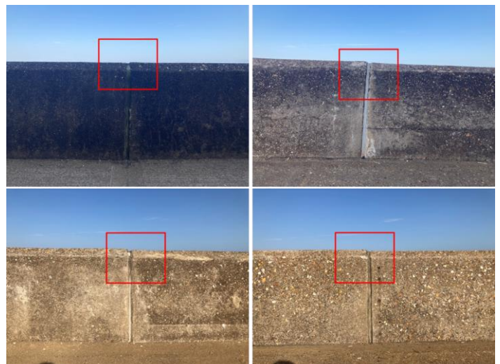
Structural movement of seawall crest
