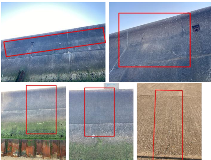
New cracking of seawall and promenade
